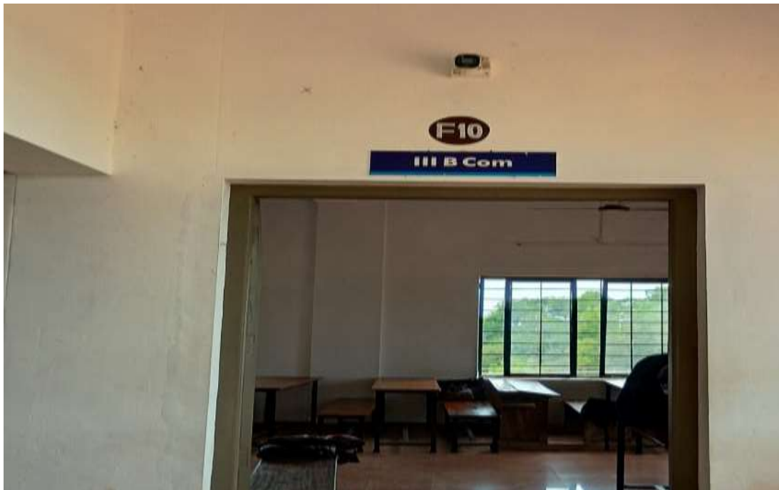
CCTV IN COMMERCE DEPARTMENT BLOCK
