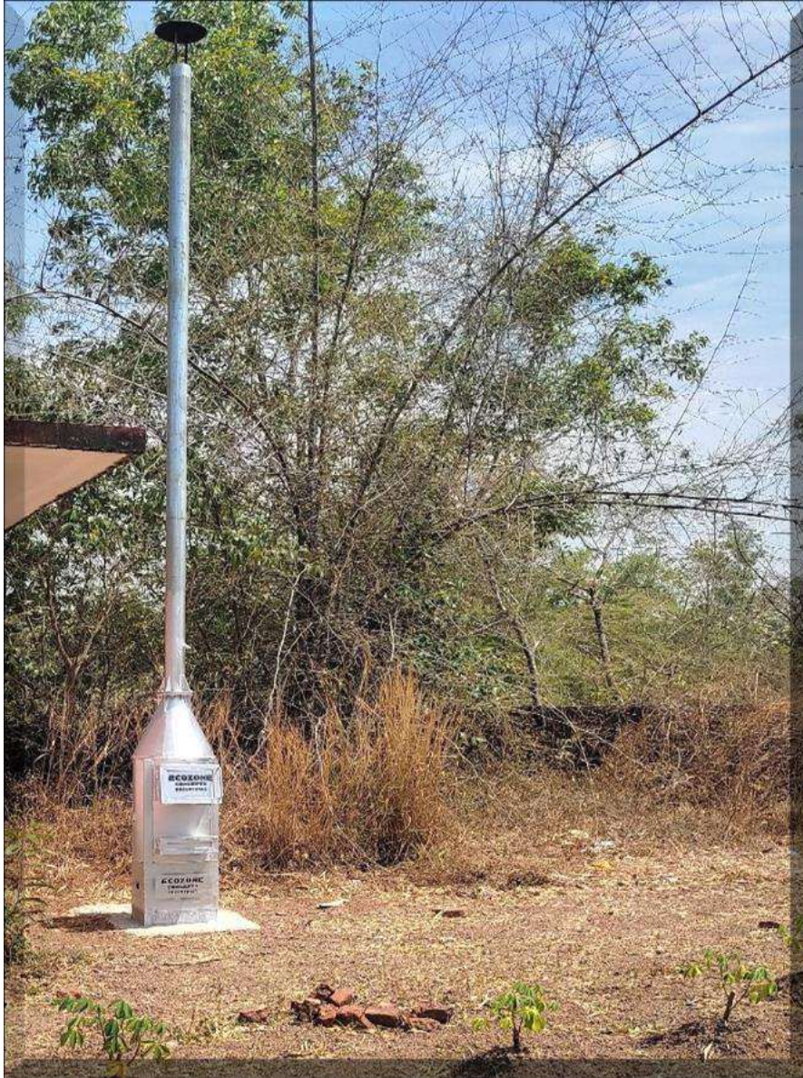
Incinerator 2 for ladies
