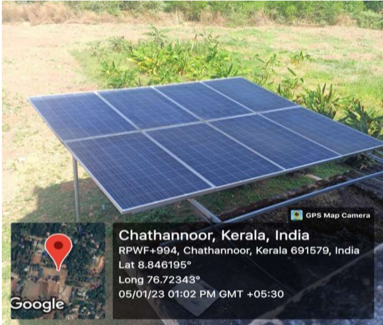
1.5 KW x 3 KV solar off grid power system installed at SN College Chathannur.
